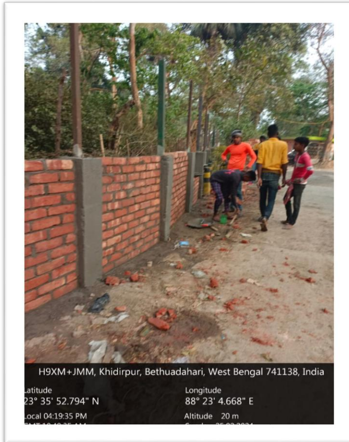
Figure 9: Brick work during development of Boundary wall and fencing at Bethuadahari Wildlife Sanctuary
